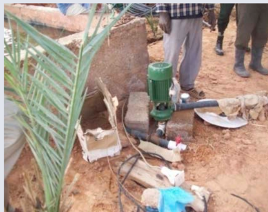
Figure 18. Installing an electric discharge pump at the exit of the storage basin for the pressurization of the localized irrigation network.
