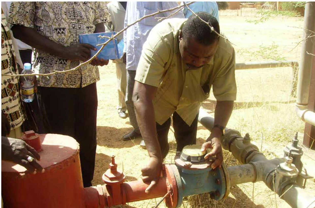
Installation hydraulique, Banizoumbou – Niger, 2007
